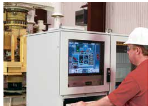
Master Control Station
